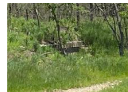
Overgrown concrete culvert on Santa Fe grade between Erie and Walnut.
